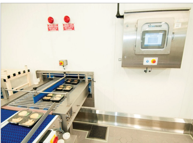
External view of Spiral Freezer infeed conveying ready meals
