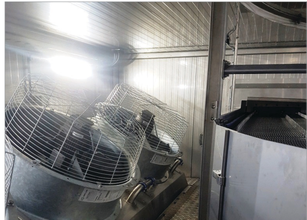
View of the evaporator inside the Spiral Freezer
